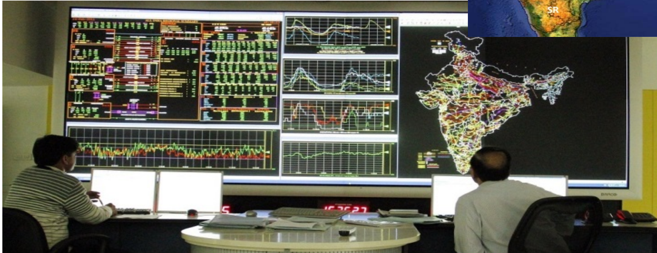
NATIONAL LOAD DESPATCH CENTER - Control room At the Top of Control Heirarchy
